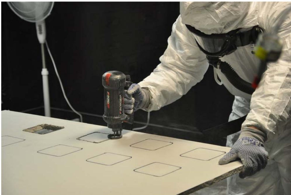
Figure 9. Cutting a 5/8” Type X drywall section with the rotary (i.e. rotozip) saw.
